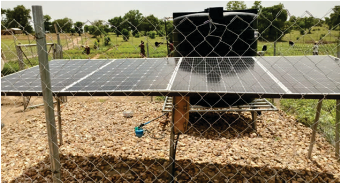
Solar mechanized borehole garden in Lore Yakin community
